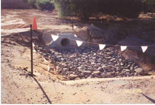
Gabion energy dissipater at an outlet. Southern Expressway
