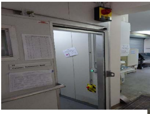
External view of cool room showing compliant internal light switch and duress button.
