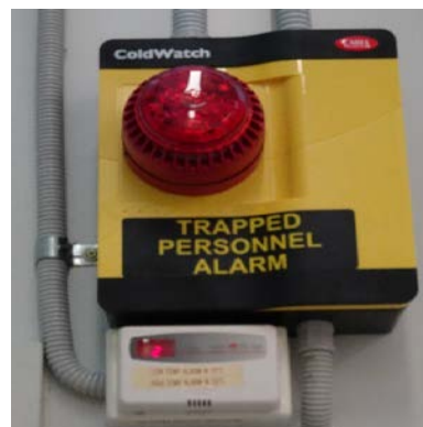
Recently retro-fitted "Trapped Personnel" alarm that flashes is located externally above the cool room door.
